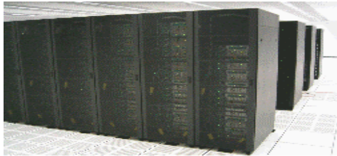
TeraGrid - Mercury IBM Itanium2 Linux Cluster 10.6 TF, 230 TB storage
